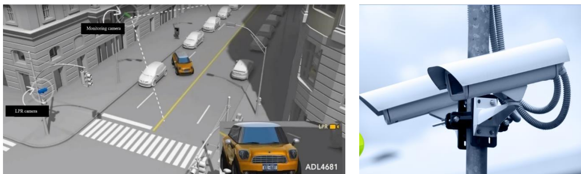
Picture 38. Examples of installed monitoring and LPR cameras on the street
