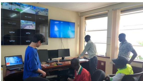
Picture 48. In the process of installing hardware at KCCA Traffic Control Center
