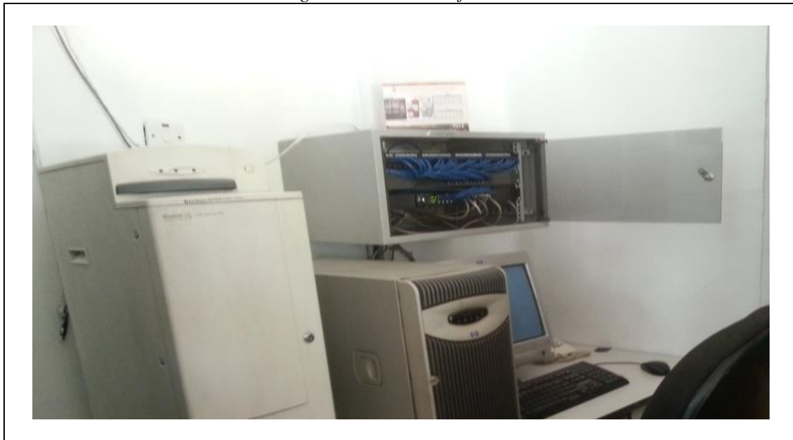
Figure III-4 Server of DCC
