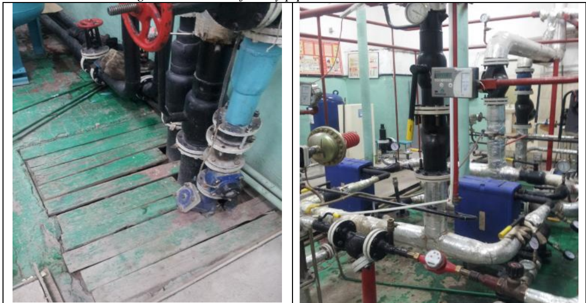
Figure III-9 Small facility pipeline in Ulaanbaatar
