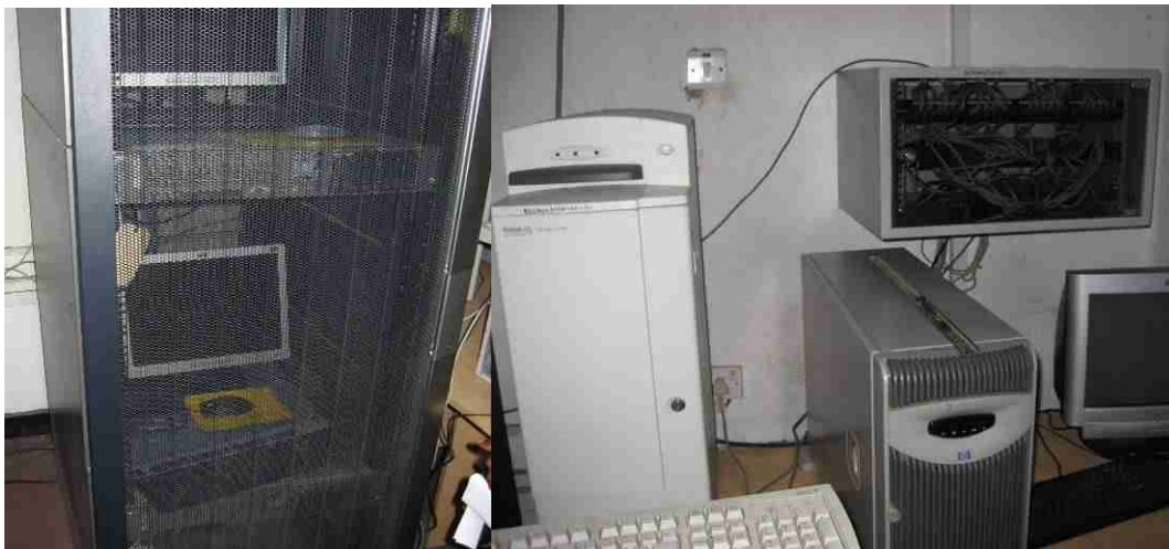
Figure 23: EPICOR Server Room
